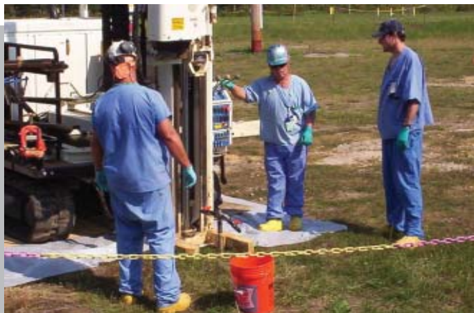
Mobile equipment is used to inject chemical oxidant into the X-701B Groundwater Plume Area to break down contaminants (primarily the industrial solvent trichloroethene or TCE).
