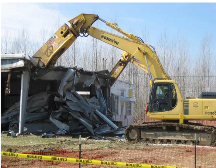
Workers dismantle the X-740 Waste Oil Storage Facility at the Portsmouth Gaseous Diffusion Plant
